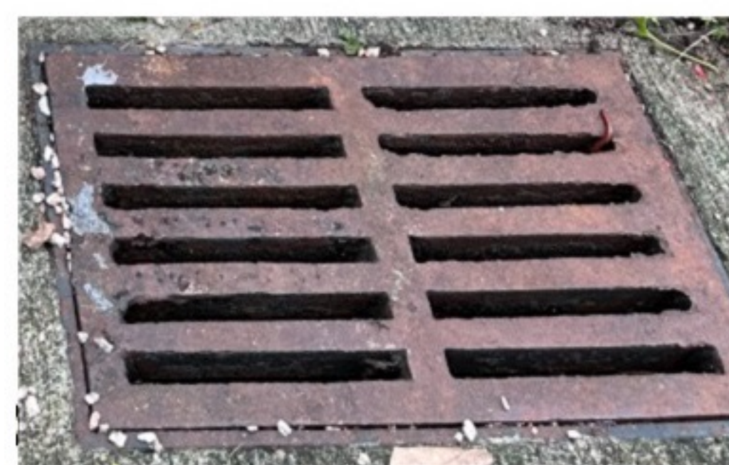
Drain outside farm on pavement
